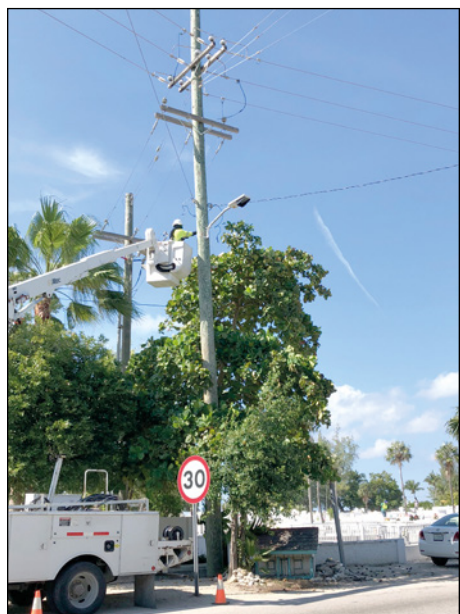
▶ CUC's Rasheed Suazo installs the first "turtle-friendly" streetlight along West Bay Road on the south side of Cemetery Beach (Photo Credit: CUC)
