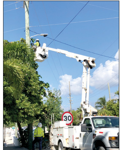
▶ CUC's Rasheed Suazo installs the first "turtle-friendly" streetlight along West Bay Road on the south side of Cemetery Beach (Photo Credit: CUC)
