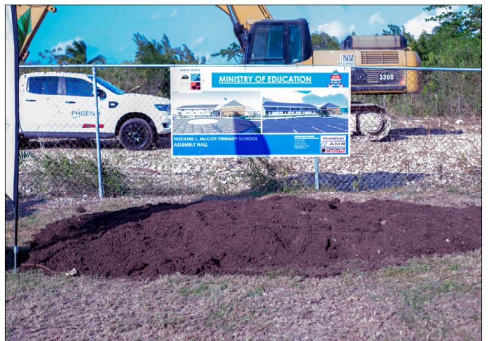
► An image of the new multipurpose hall to be constructed at the Theoline L. McCoy Primary School.
