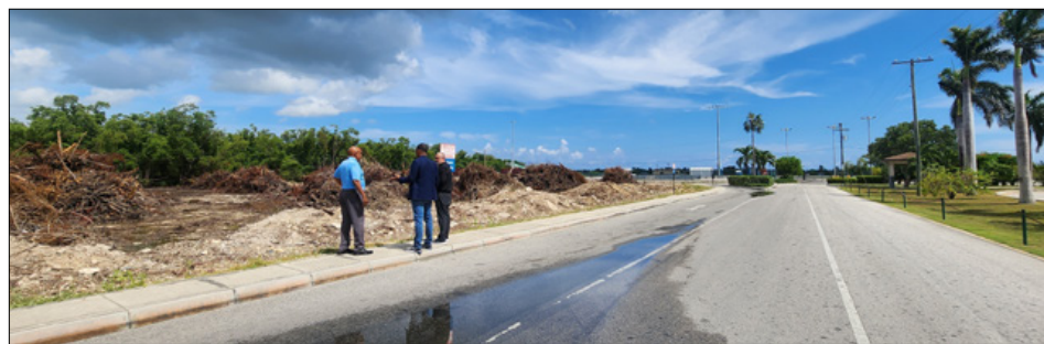
► CIAA CEO Albert Anderson, Minister for Tourism and Ports Kenneth Bryan, and CIAA Board Chairman Johann Moxam visit the site of the new parking facility
