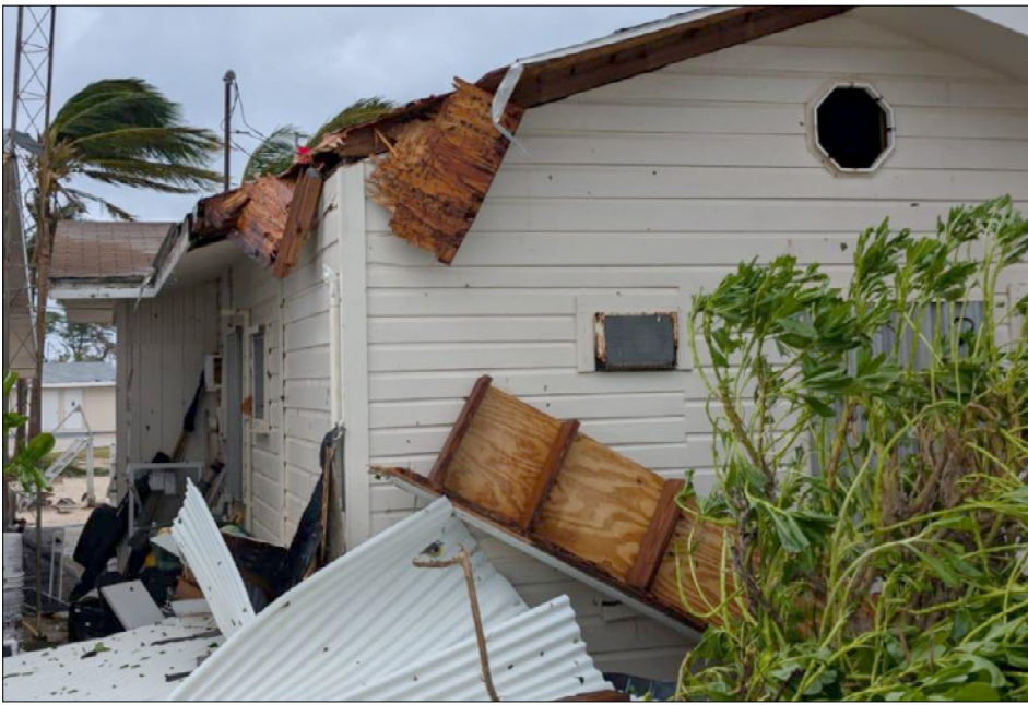
► Property damage on Little Cayman caused by Hurricane Rafael
