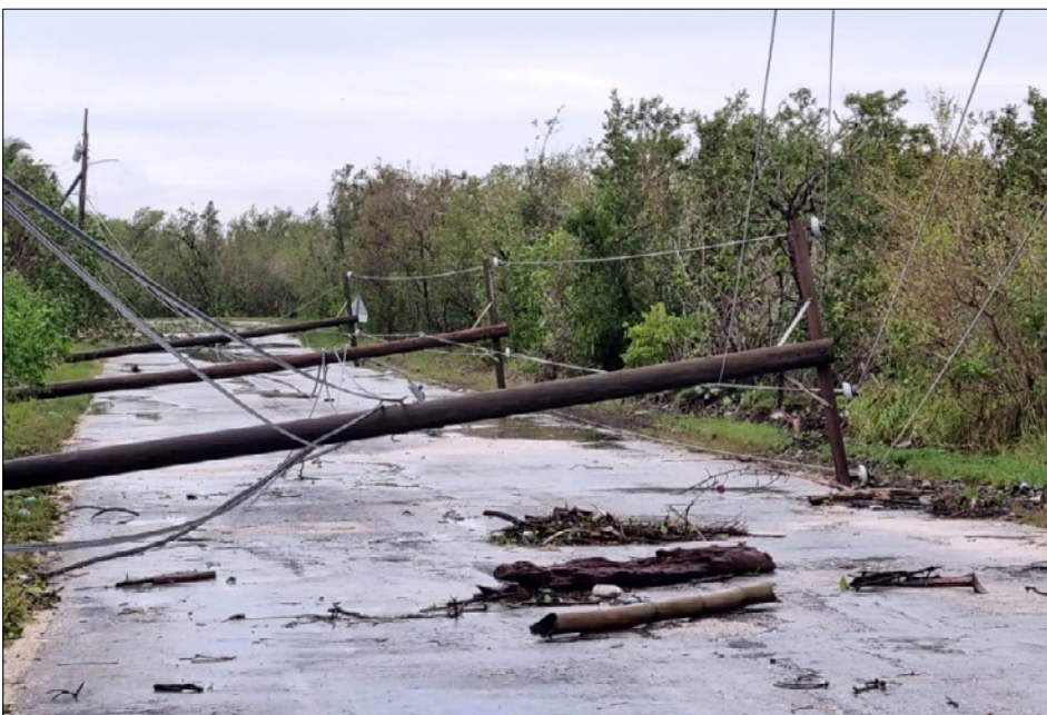
► Downed poles and cables block road
