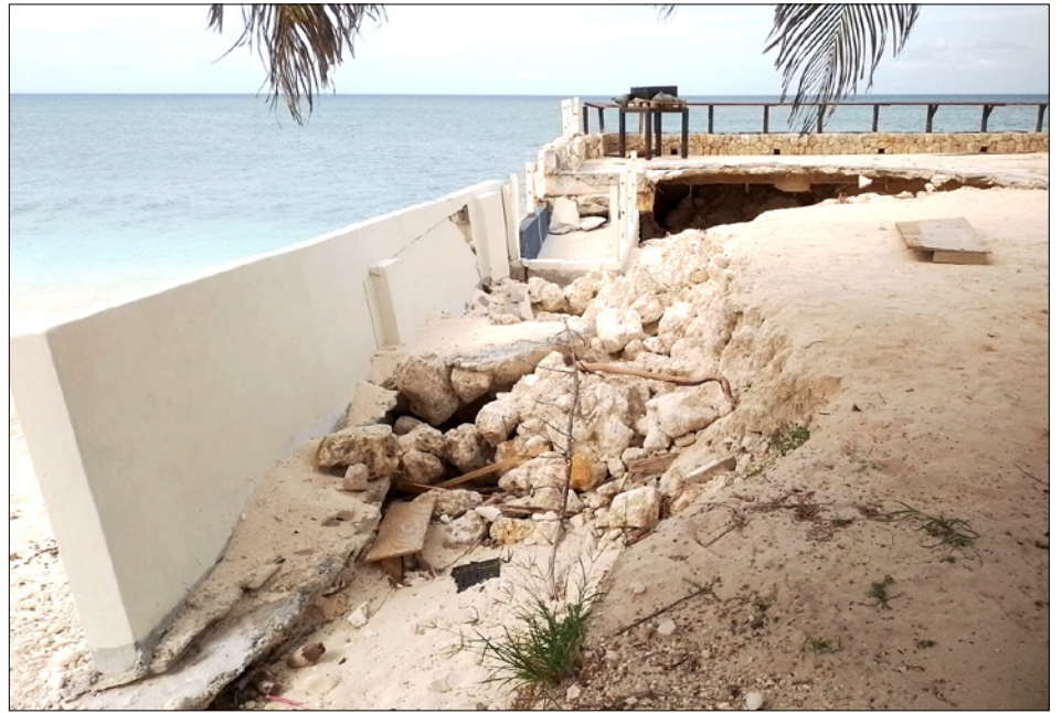
► The Area in which the building was formally housed continues to create a large man hole with the passing storms of hurricane season
