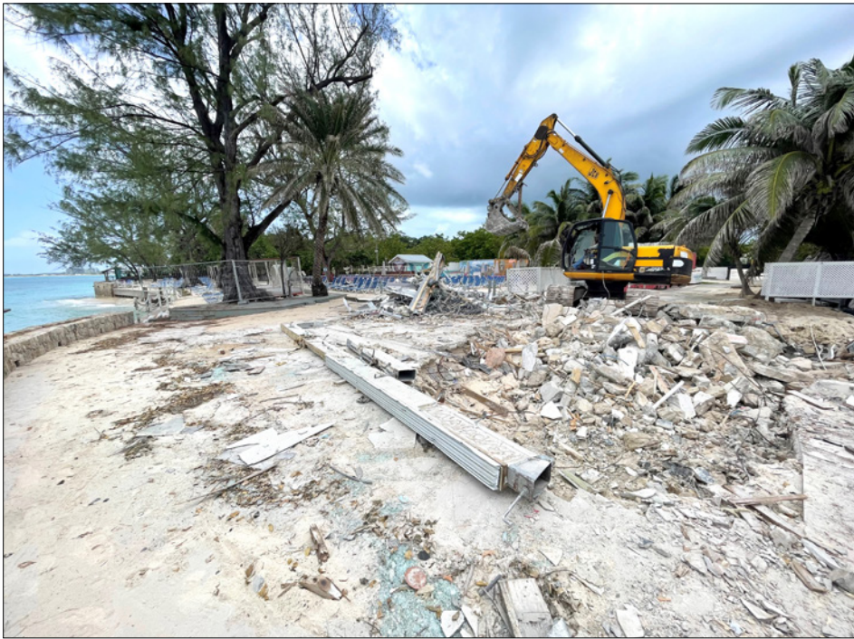
► The main bar building was demolished in the summer of 2024, following severe storm damage in February 2024 which resulted in the building being condemned.
