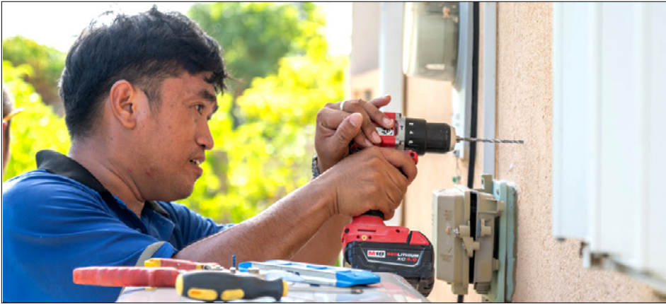
► A Parsons AC Technician installs a new energy efficient unit at a private home
